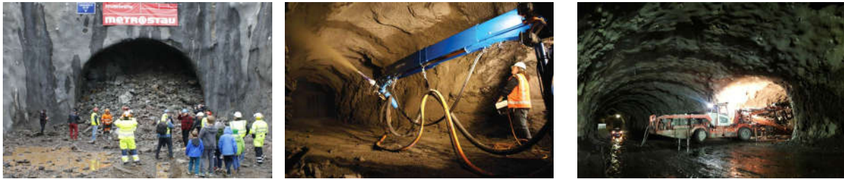
Figure 1. Tunnel work documentation: a) tunnel front secured by sprayed concrete, b) example of the sprayed concrete device, c) tunnel drilling works.
