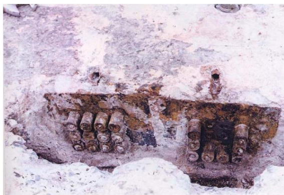
Figure 5. Corroded top slab anchors – some barrel grips completely corroded away
