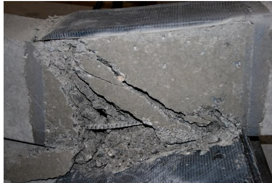
Figure 5-17. Crack pattern of BSb6 at ultimate load.
