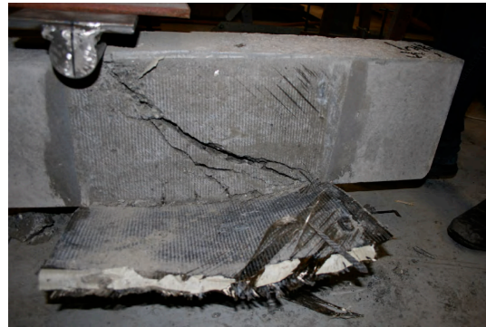
Figure 5-10. Crack pattern for BSa8 at ultimate load.
