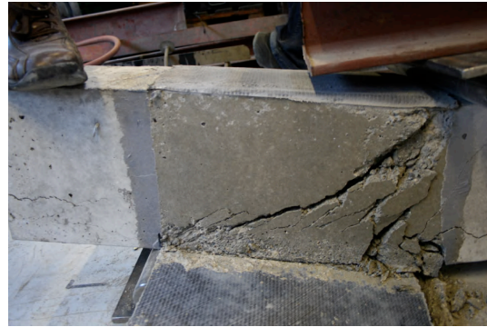
Figure 5-14. Crack pattern for BSb4 at ultimate load.
