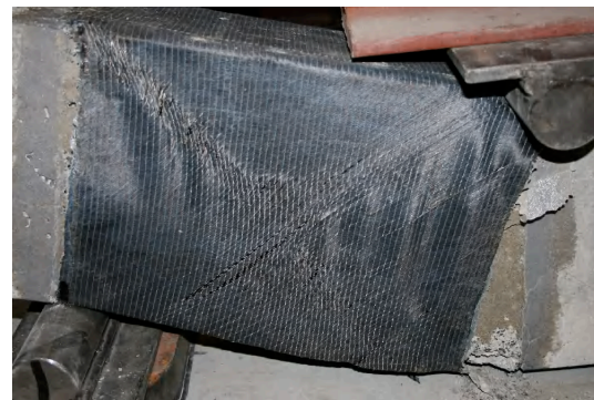
Figure 5-16. Rupture of BFRP sheet on BSb6.
