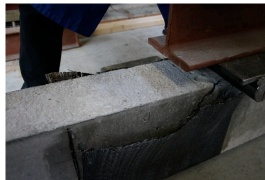
Figure 5-6. Bond failure, BSa4.
