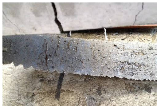
Figure 5-26. BFc9 (EPOXY1), de-bonding of BFRP.
