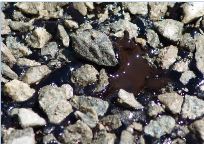
Figure 16 - 10 minutes after aggregate application. Binder has started to cure as can be seen on the black film and the brown color underneath the stone that was removed. Choke stone was not applied until 5 minutes later.
