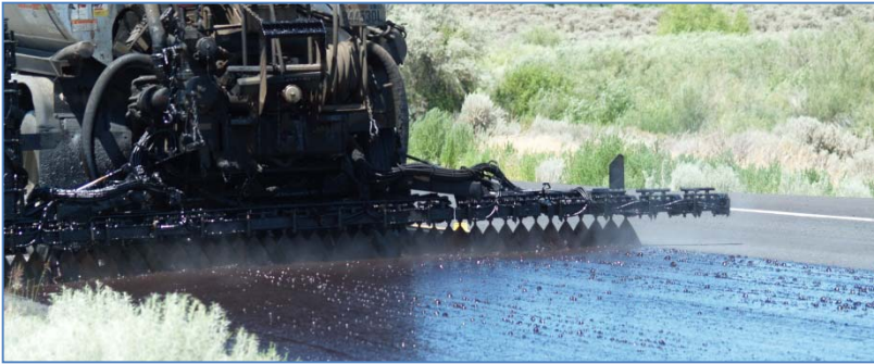
Figure 38 - Project visit 7.7.2009, streaks in the asphalt binder will cause corn rowing
