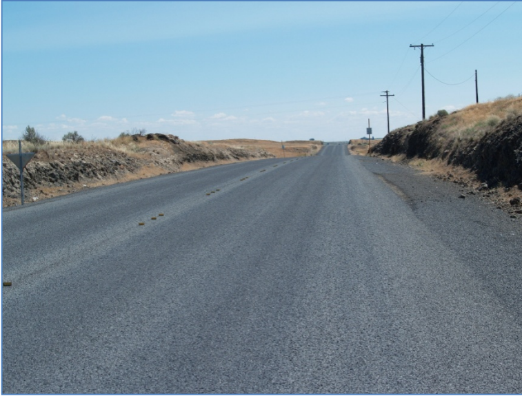
Figure 31 - 1 day old chip seal. The section had been swept and looked good.
