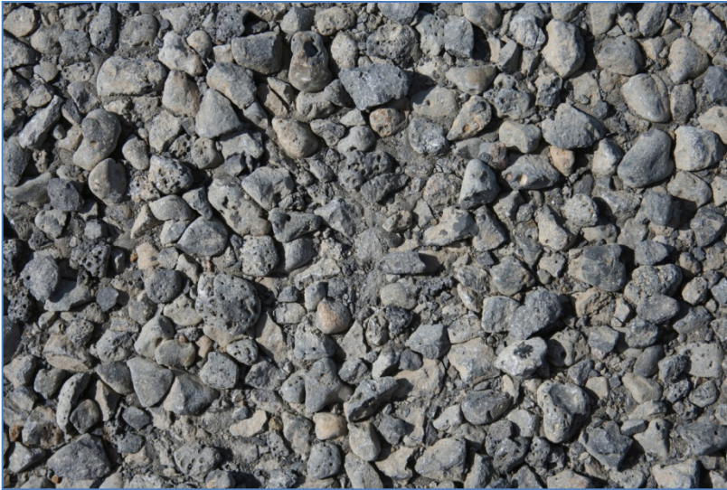
Figure 41 - Rough textured existing surface
