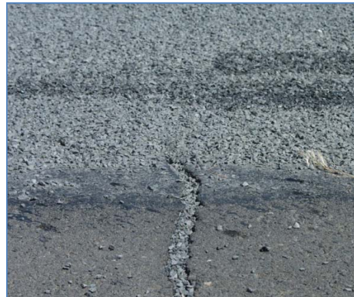
Figure 33 - Transverse 1.5 inches wide unsealed thermal crack. The crack is visible through the chip seal applied the previous day
